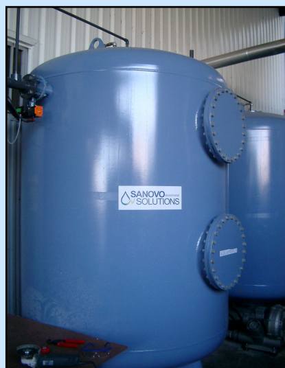
Arsenic removal plant
