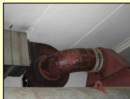
A typical hot air pipe as it appears to you.
